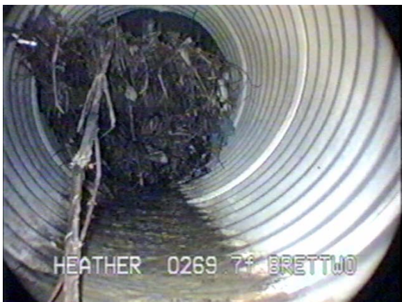
A blockage clogs this storm sewer
