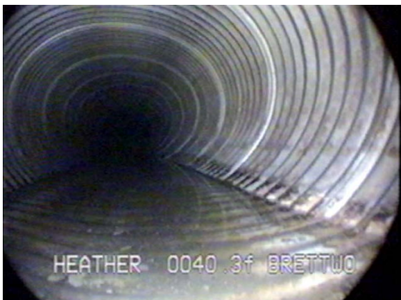
This storm sewer is clean and working properly
